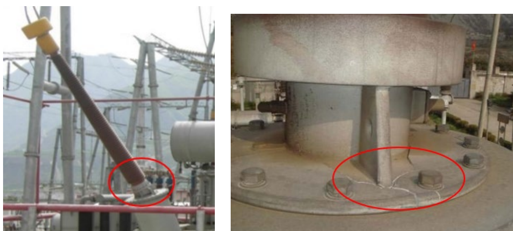
(c) 套管法兰断裂
