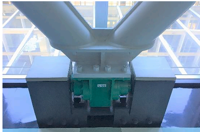
Fig. 7. Intact novel oil damper brace.
