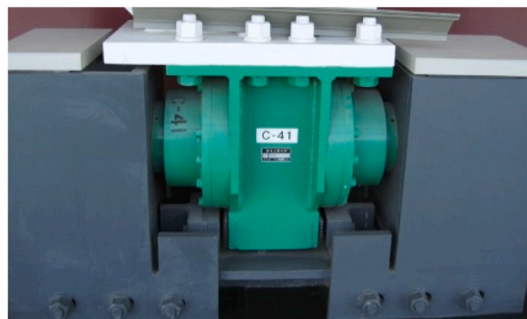
Fig. 5. Intact oil damper.
