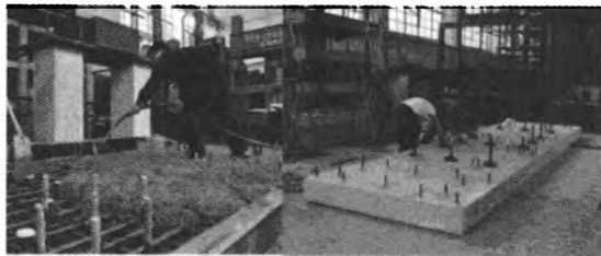
图6 塔线体系刚性底座设计 Fig. 6 The concrete base for tower-line coupling system
