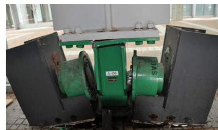
Fig.6. Damaged Oil Damper and Abutment
