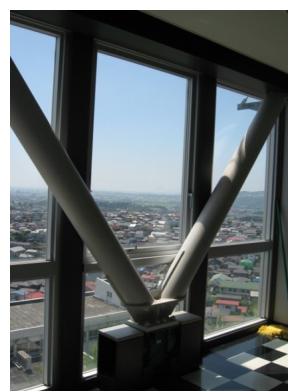
Fig.3. Brace of the Oil Damper
