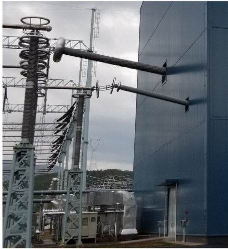
Fig. 1. \pm 800 kV UHV wall bushing mounted on a gable wall.
